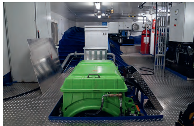
Engine room aft with Oswald electric motors.
