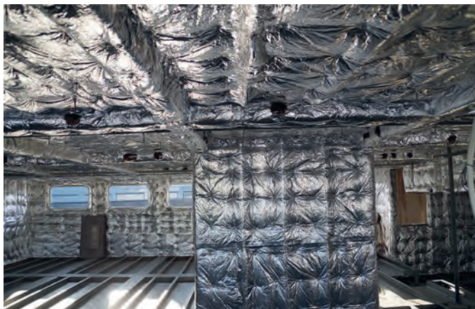
The aft deckhouse without gangways is highly insulated. This results in low decibel measurements.
