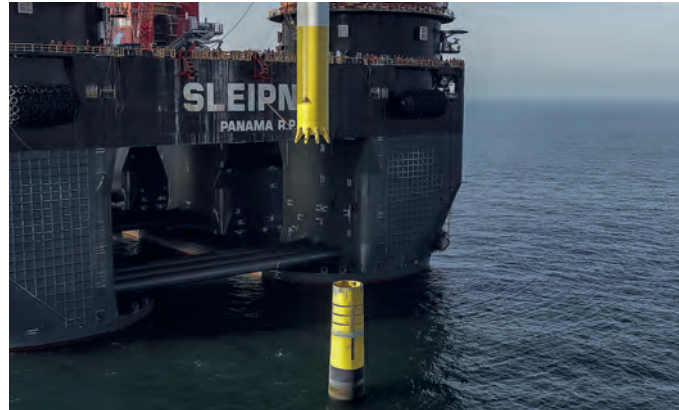
DOT's Slip Joint connecting the wind turbine's lower tower to the monopile foundation (photo TU Delft).
