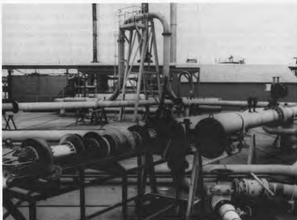
fig. 7: 16 in. RPIT in front of launch/receive trap of 16 in. testloop located at Shell laboratories
