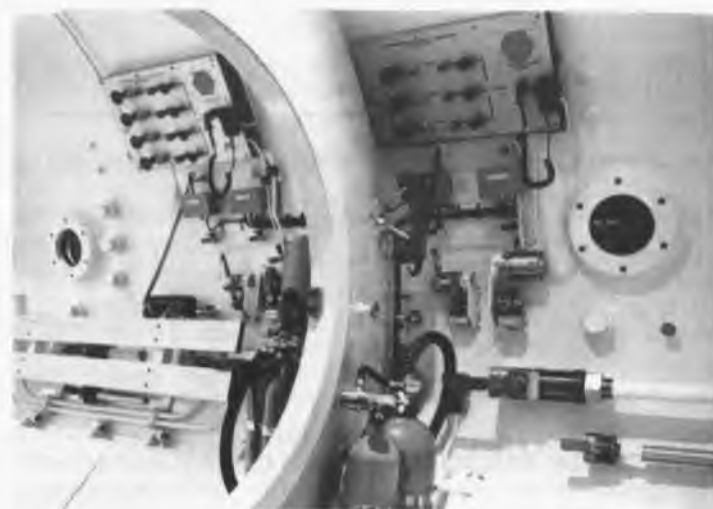
The interior with oxygen/mix-gas panels.
