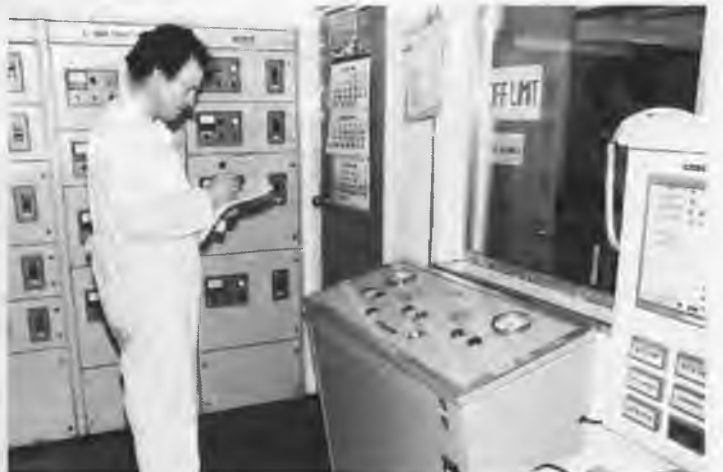
The 'Emulsa' control cabinet in the engine control room of the Bell Ruler.
